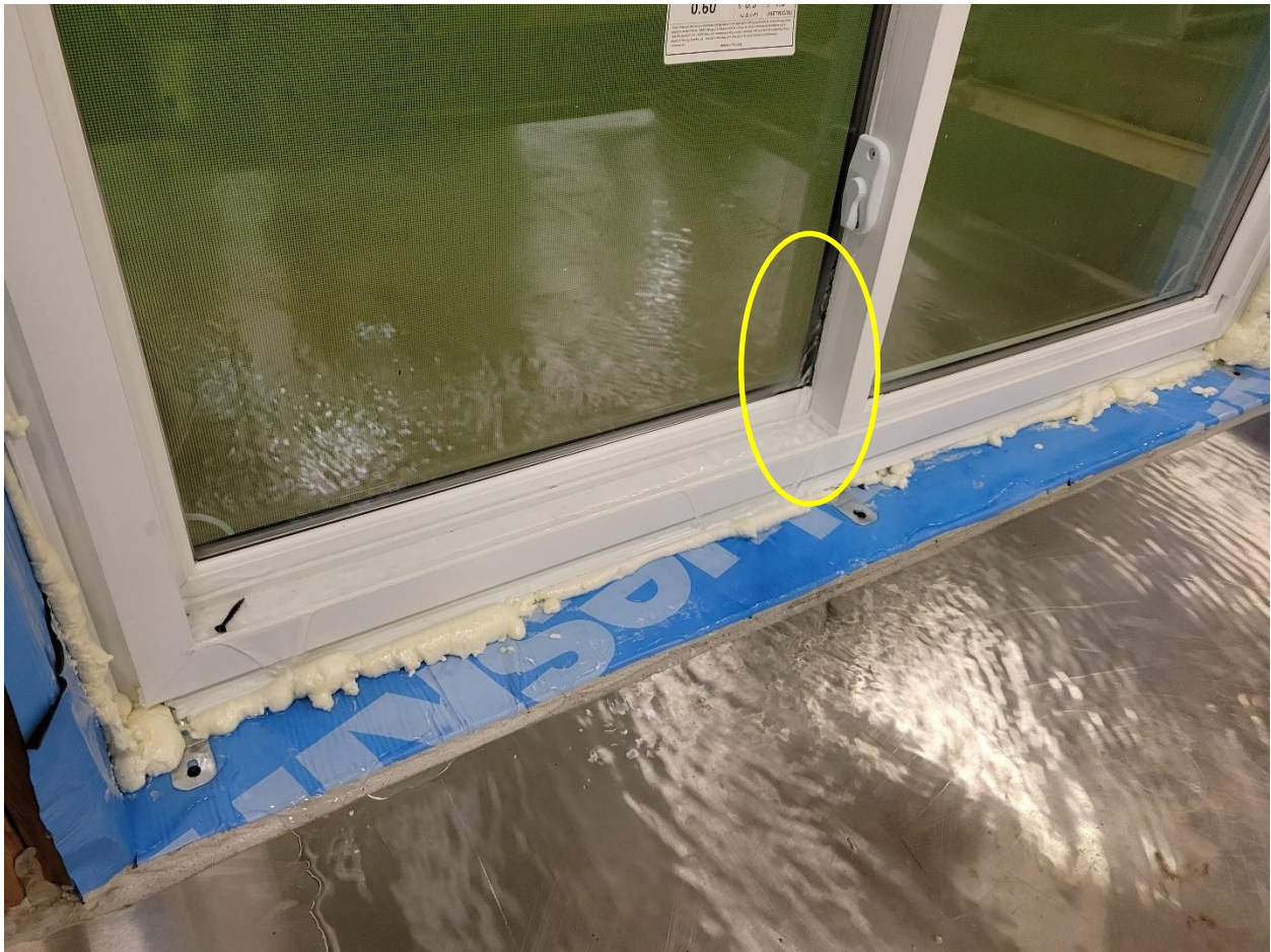
Figure 44. Leakage observed between the two panes of the sliding window in the MWB.
