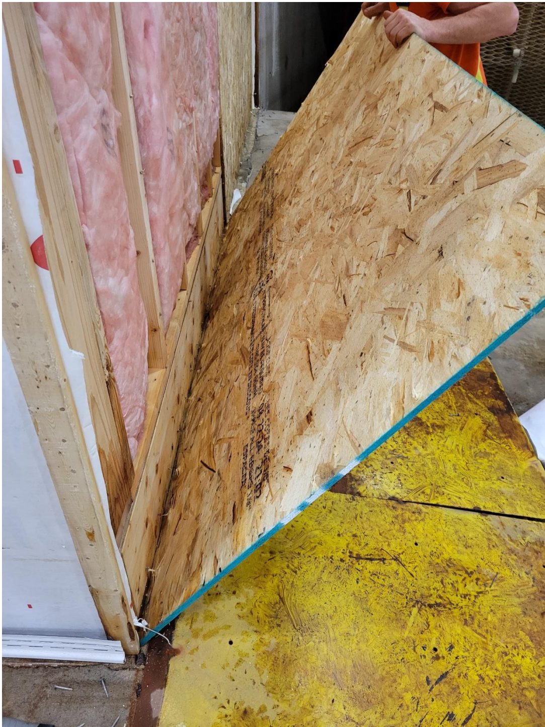
Figure 37. Water damage between the rim joist and the exterior plywood sheathing in Phase 1.
