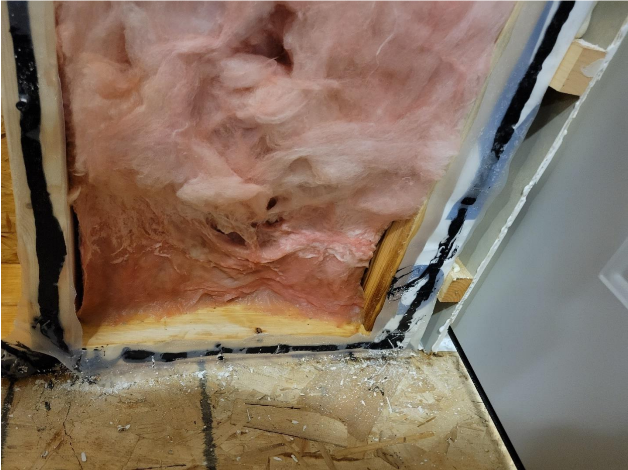
Figure 38. Saturated fiberglass insulation found just beside the door during the deconstruction after Phase 1 testing.
